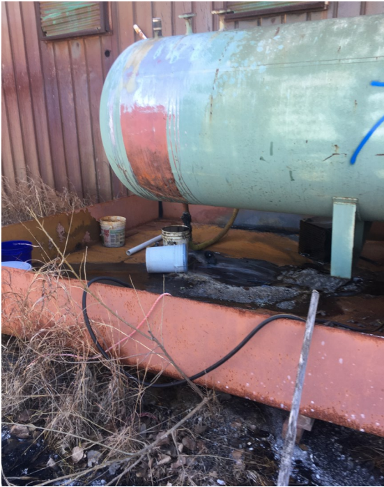
Leaking end of Tank #1
